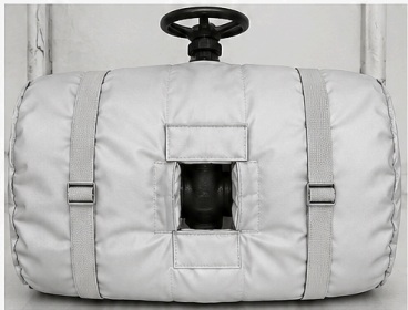
INSULATED SYSTEM IN THE FIELD
